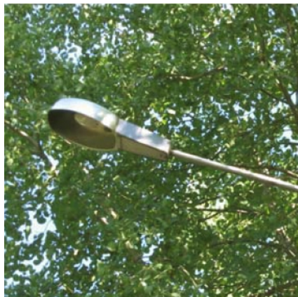
Figure 39; Example of functional luminaire IP21 that was excluded from this improvement option, reason: the open optic has a poor LMF due to dirt.
