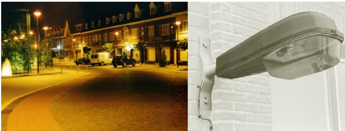
Figure 19: Street lighting luminaires attached to poles(left) and to a house (right)
