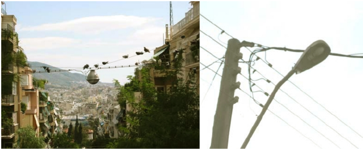
Figure 18: Street lighting luminaire attached to cables(left) and to electricity distribution (right).
